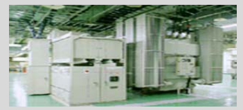
Power supply systems
