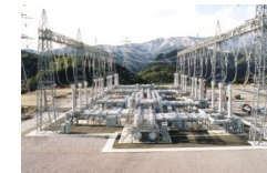
Gas Insulated Switchgear
