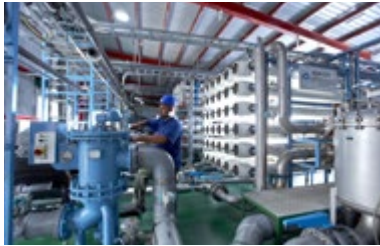
A seawater desalination system.
