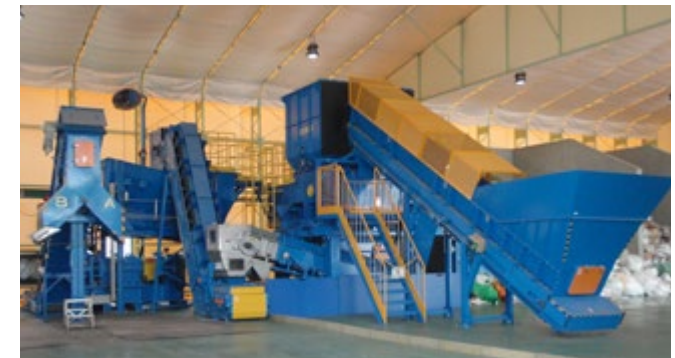
An RPF manufacturing facility.
