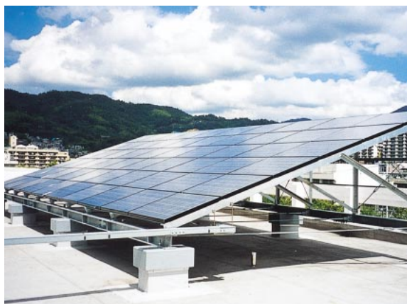
Solar Power Generation System (Kure Technical College)
