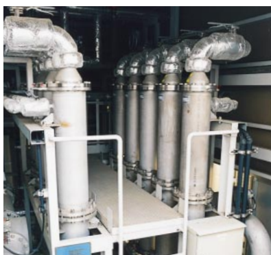
Using a membrane filter, this wastewater treatment device at Hitachi's Naka semiconductor production facility plays a crucial role in the recycling of wastewater.
